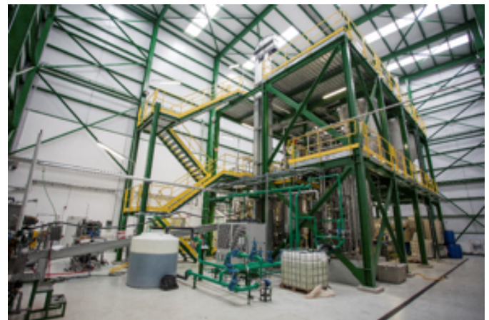
Figure: BIO2C demonstration plant (CENER).
