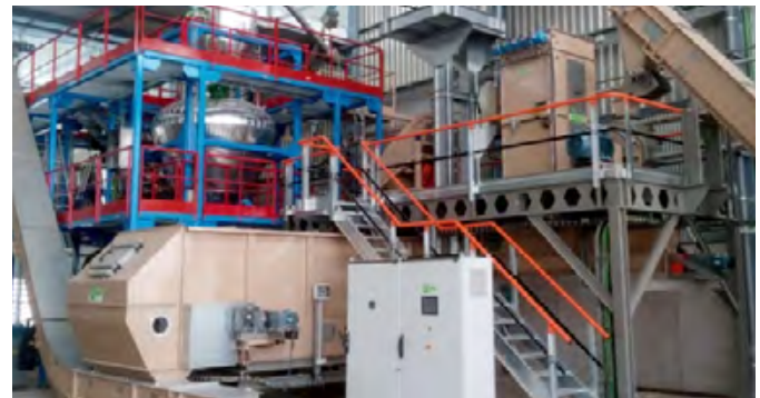
Up-stream unit of the lignocellulosic biomass
