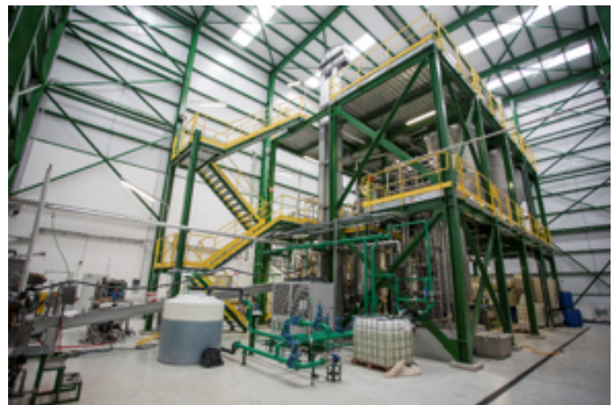
Figure: BIO2C demonstration plant (CENER).
