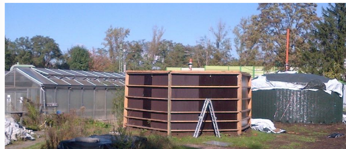
Figure 2. Construction of a prototype with modular wall elements in wood construction (still without panelling). In the background: The three-aisled greenhouse to be heated and a round Compost heater made of double-bar fence elements with horizontal heat exchanger.
